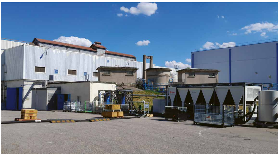
Papeteries de Clairefontaine - refrigeration unit and heat exchangers
