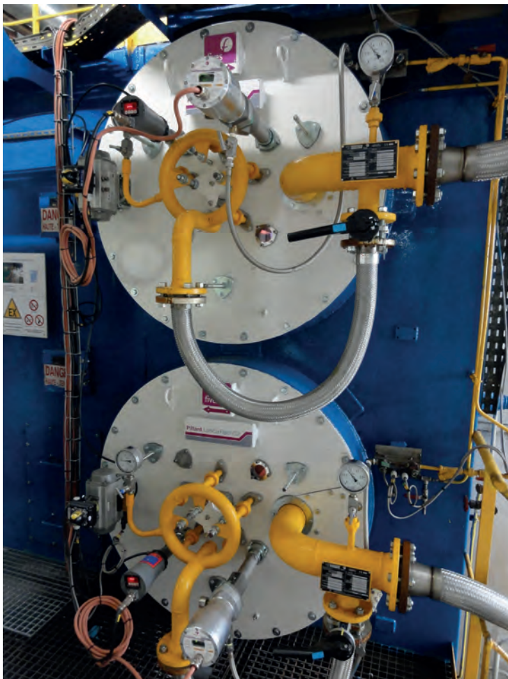
New low-NOx burners on one of the Papeteries de Clairefontaine boilers.
